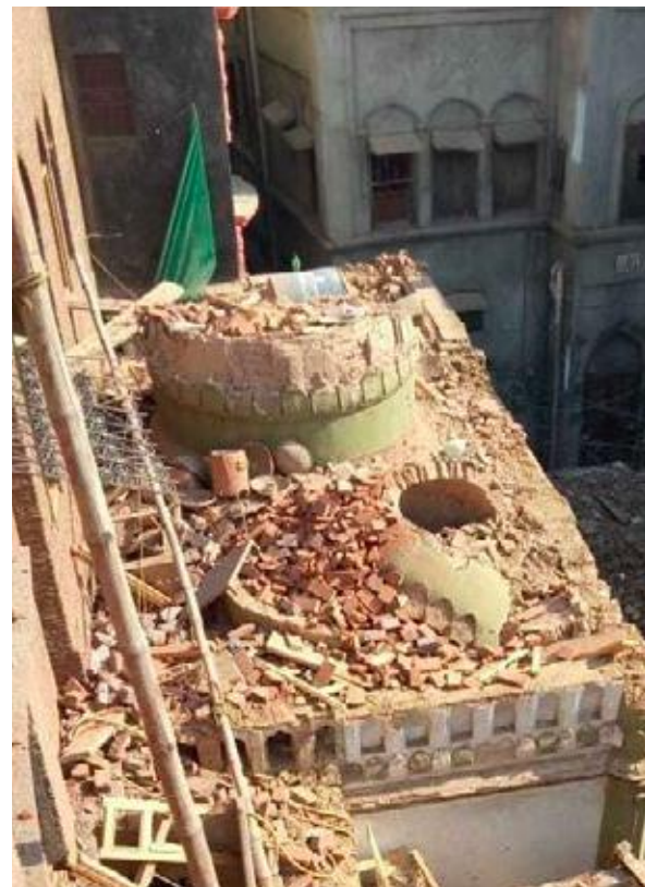
Demolished minarets of Sialkot Mosque
